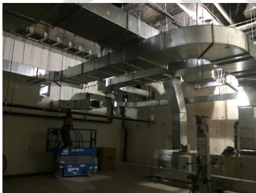
Figure 5.9 Ductwork in a mechanical room
