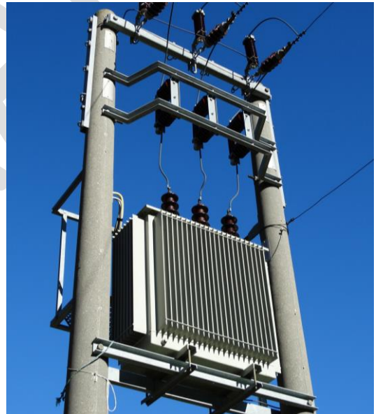
Figure 7.16 Pole-mounted distribution transformer
