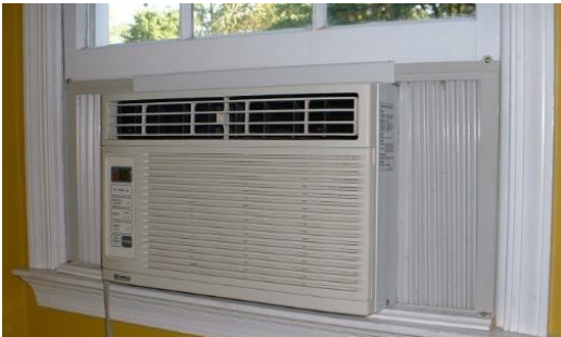
Figure 5.4 Window air conditioner
